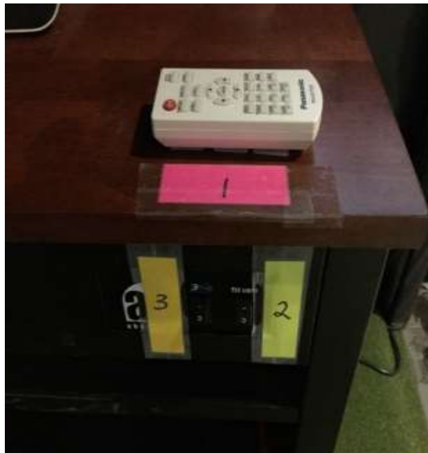
Switches #2 and #3 turn on Tee Light and Monitor
